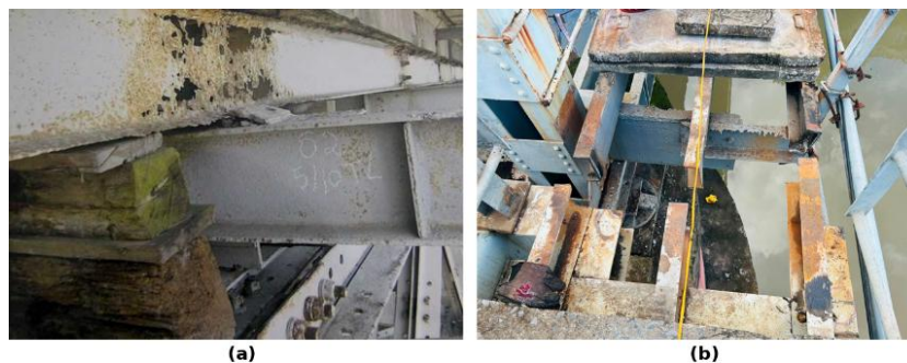
Figure 1. Typical damage of steel girders in railway bridges: (a) web perforation and rivet-hole perforation at the flange (source: Bao Xay Dung [3]); (b) corrosion of the top flange causing area loss at Tam Bac bridge, Hai Phong (source: Bao Cong Ly [6]). The press sources [3,6] document the occurrence of the damage only, not technical data.
