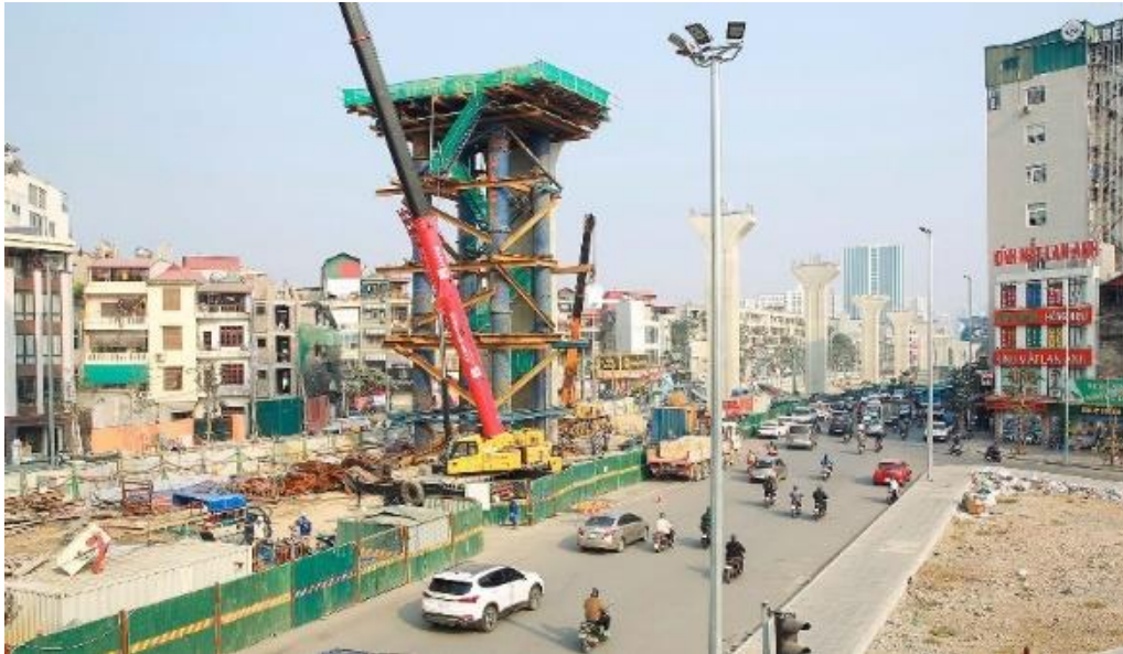
Figure 1. Ring road no.2 during construction (The picture was taken on 10 th April 2022 by authors)
