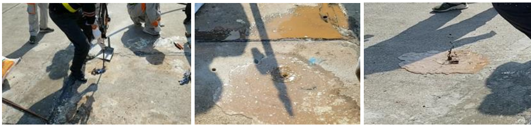
Figure 7. Water and mud pumped out from foundation-subgrade of rigid pavement while applying treatment solution of polyurethane injection at tested location at NIA's apron.
